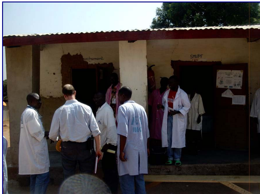
The maternity ward prior to rehabilitation
